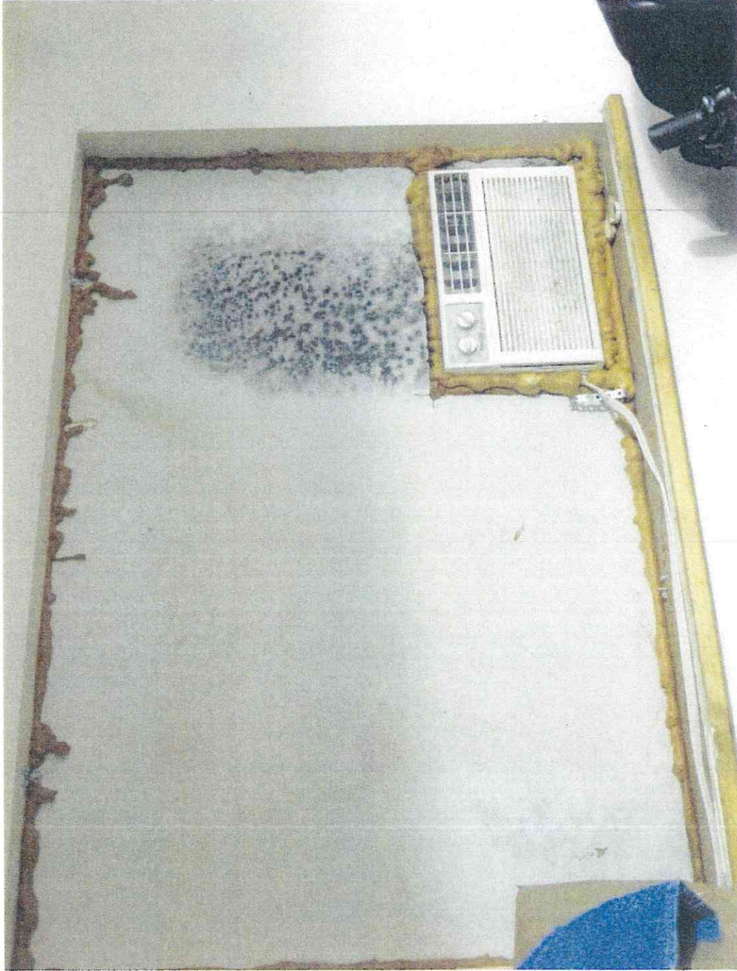
A window inside the residential MMAR production site was boarded up and sealed with spray foam. Mold was growing on the wall inside from the extensive use of the air conditioner.
