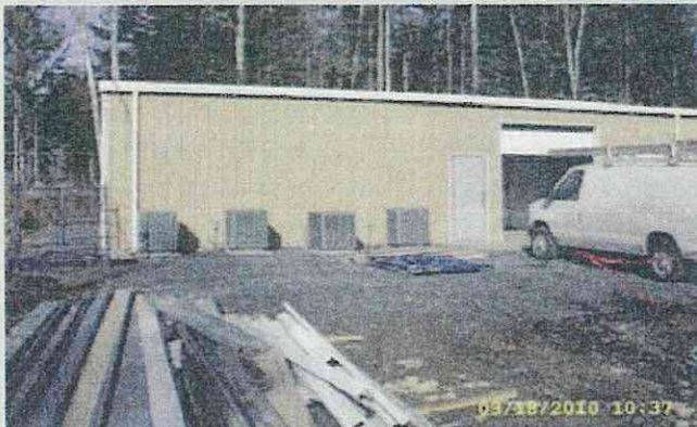
There were nine air conditioning units outside (four visible in this picture).
