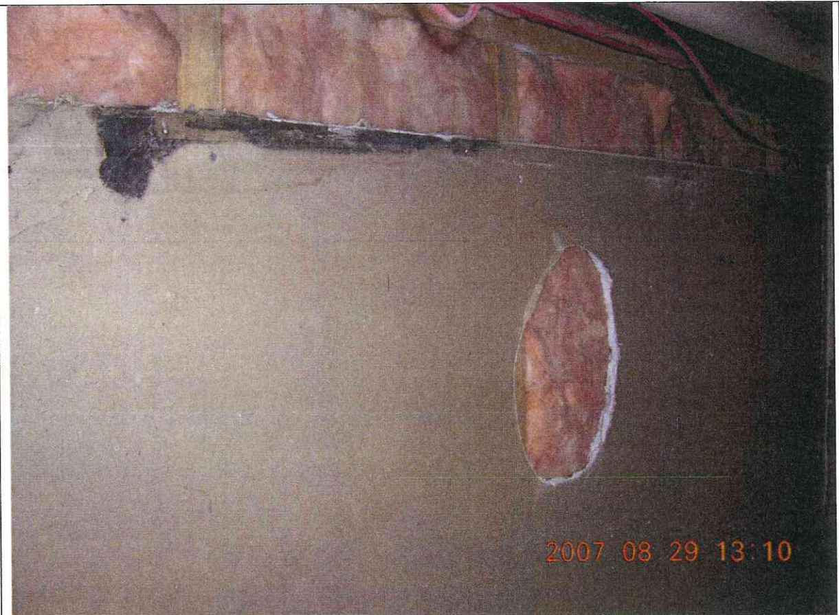
Photo 2 Example of: Minor Mould Growth (1) Description: This photo shows an example of minor mould growth (dark staining on top left corner of drywall). Minor mould growth is to be considered <math>< 1\text{m}^3</math>.
