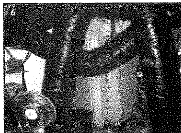
(6) Flexible ducts, used to exhaust telltale odor and circulate air, pose a common entanglement hazard in most grow houses. [Photos courtesy of Miami-Dade (FL) Fire Rescue.] (7) This grow house partially collapsed as the result of an explosion caused by propane leaking from a cylinder. The propane fueled a carbon dioxide generator.
