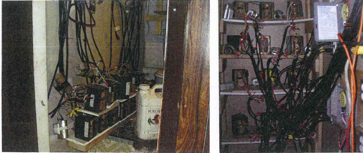
Examples of electrical issues found in MGOs with children.
