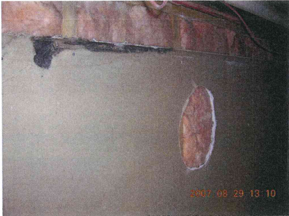
Example of minor mould growth (1)
