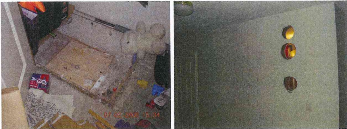
Examples of structural issues found in MGOs with children.
