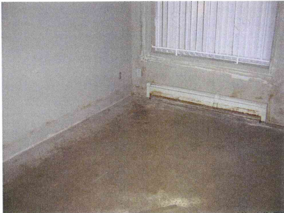
Example of suspected mould growth (S)
