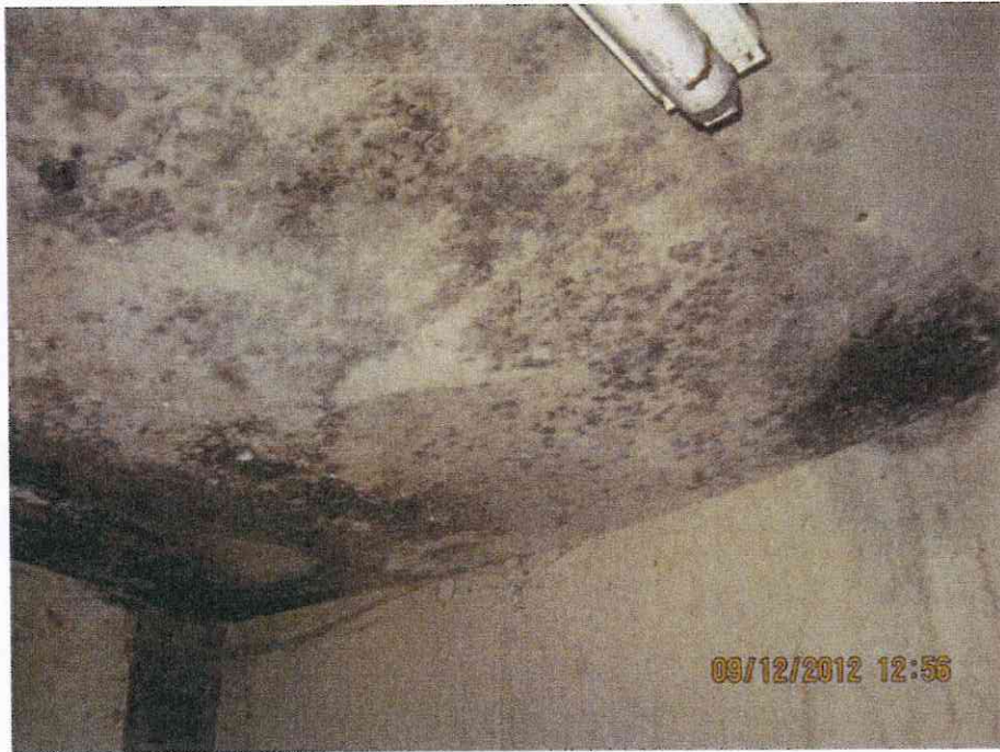
Example of major mould growth (2)
