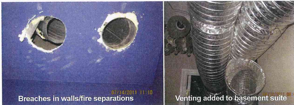
Examples of unsafe building modifications found in MGOs.
