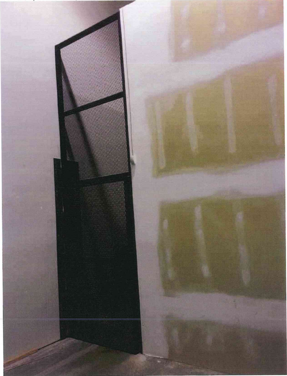
Steel Security Door & Wall System w/ Enclosed Pad-Lock (Rear):
