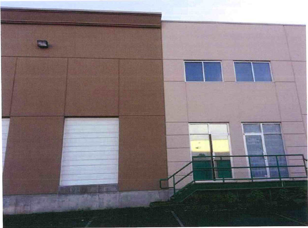
Rear: Exterior Door Fitted w/ Heavy Gauge Steel Anti-Pry Plate
