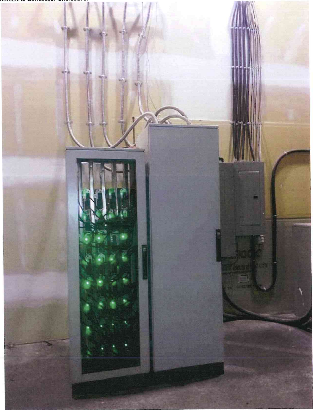
Ballast & Contactor Enclosure:
