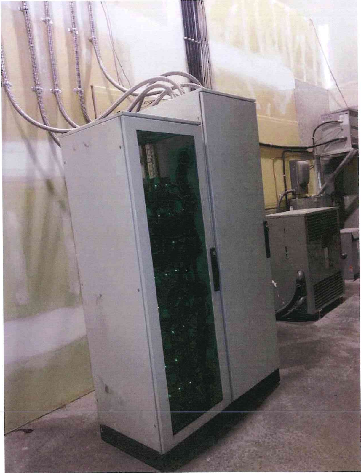
Power Distribution Area:
