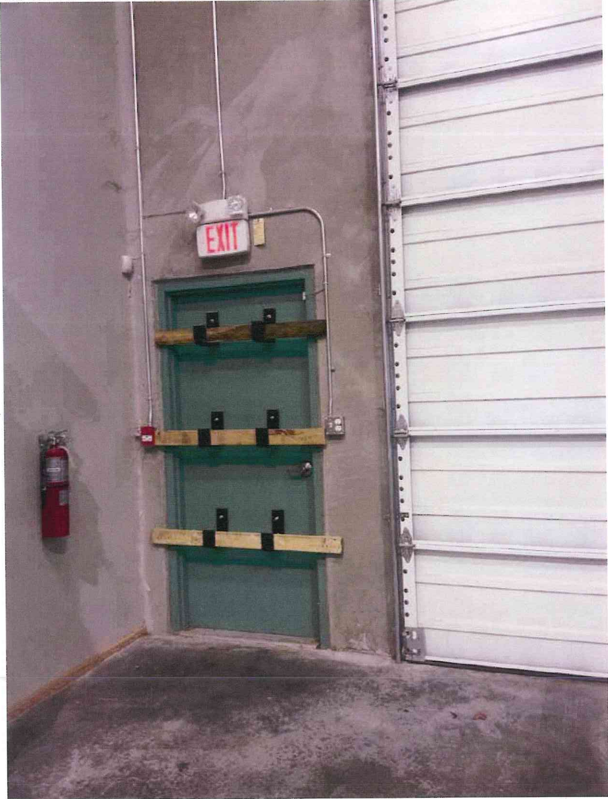
Exterior Man-Door: Located at the front of building (Photo taken from interior):
