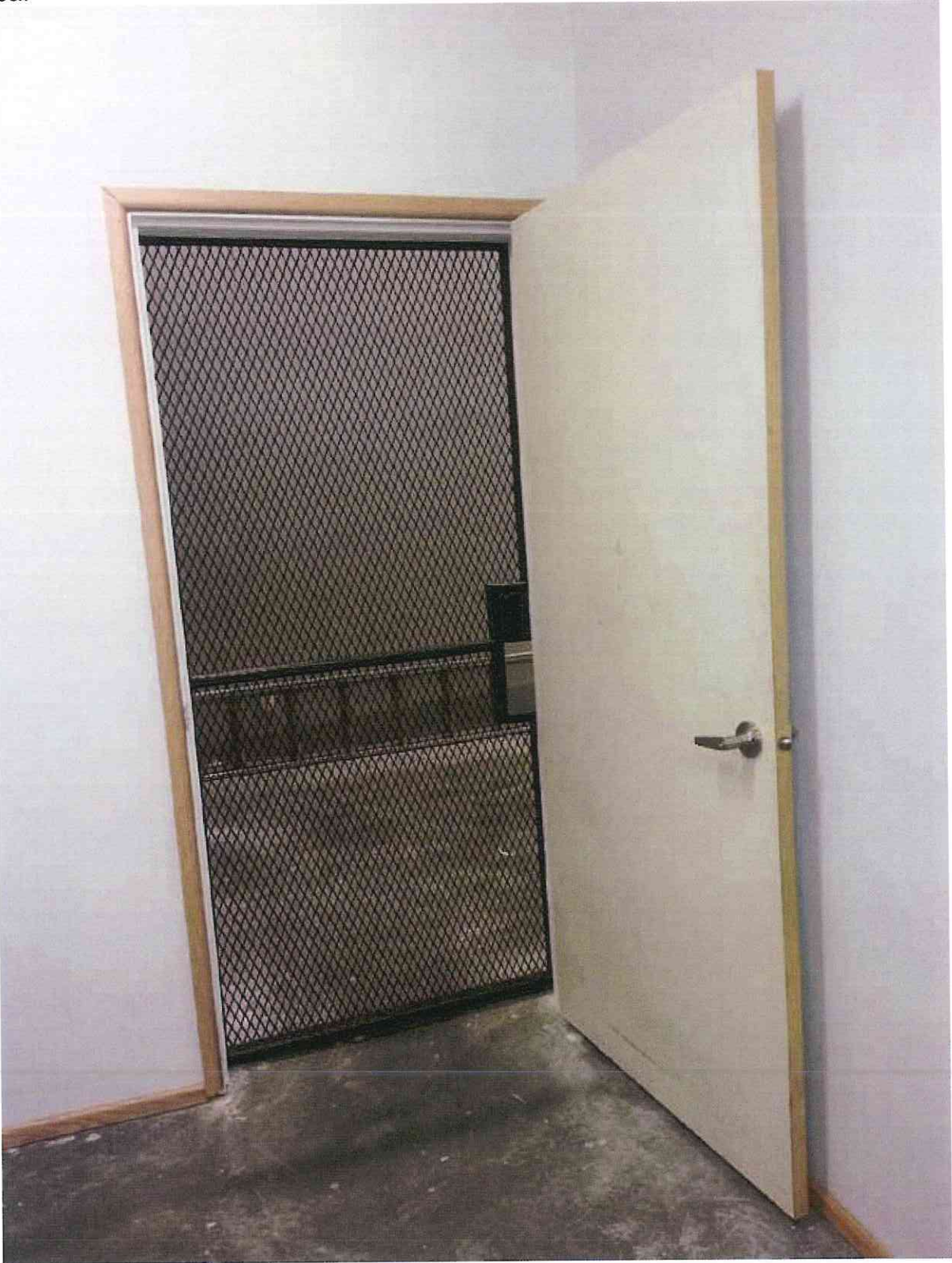
Front Office Interior Door w/ Keyed Locking Handle & Additional Steel Security Door w/ Enclosed Pad-Lock
